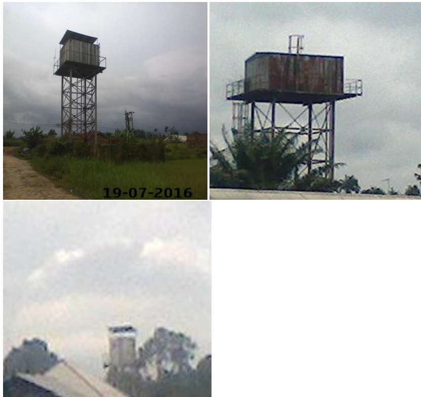
Plate 4.5g: pic 1-2 (Water facilities at Odorubu community); pic 3 (the only water facility at Lalagbene community) which ought to be providing potable water for inhabitants but no longer functional.
