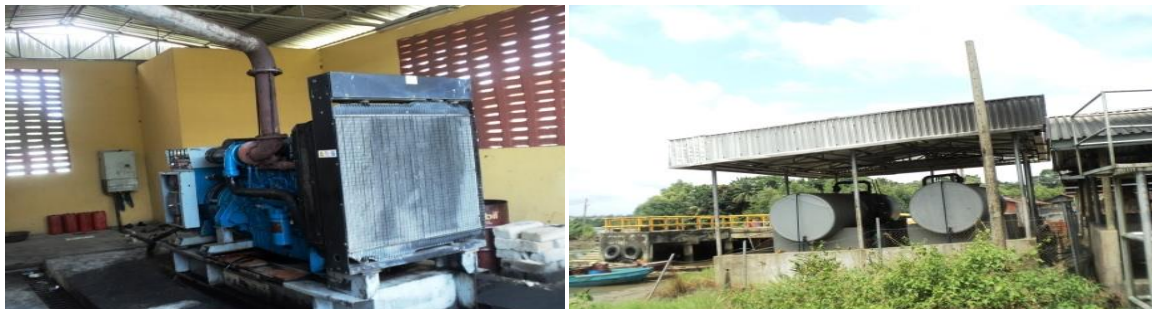
Plate 4.5b: Two giant generators supply electricity to the project communities
