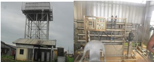
Plate 4.17: The Community water facility and with its water treatment facility
